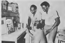
at far right among an array of pneumatic and electronic control instruments. The CMA is the latest development in Direct Digital Computer control.
